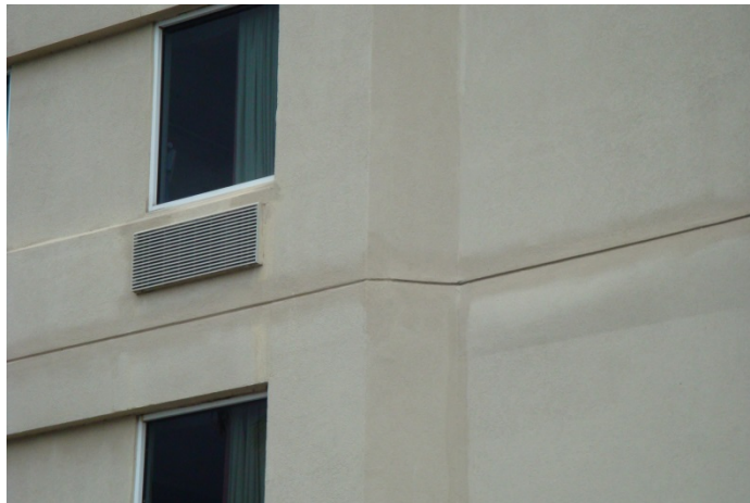
More Water Penetration
