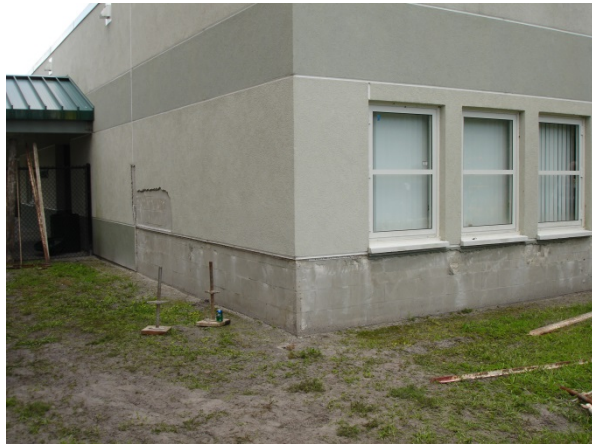
Deer Park School - More Stucco Repair
