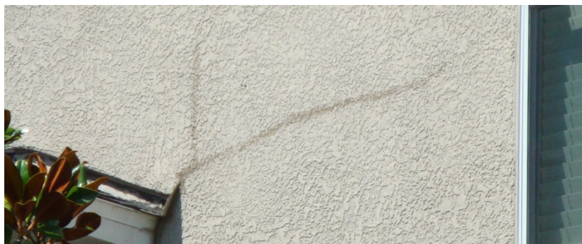
Hydration Cracking with Water Penetration
