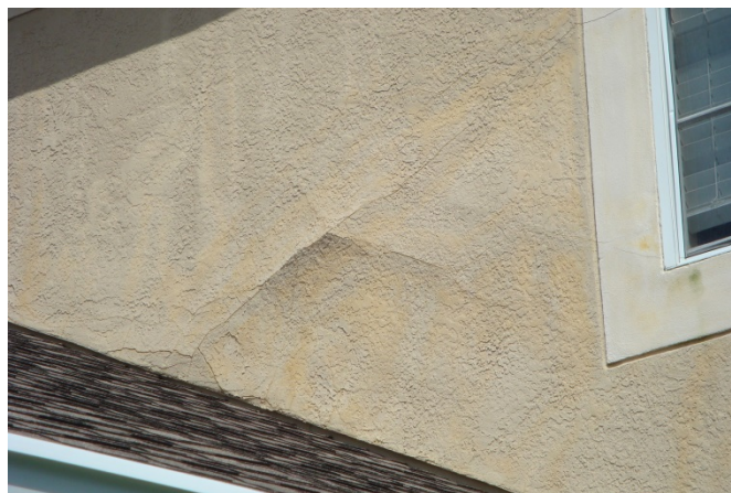
Delamination from water penetration
